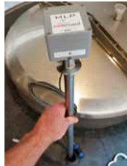
The MLP on top of the tank.
